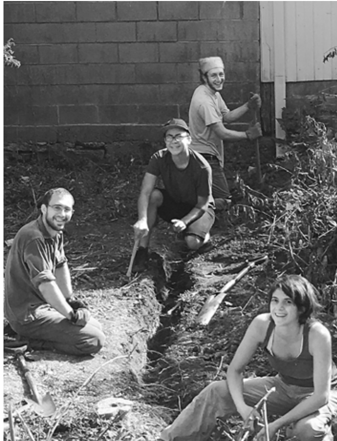
Helping dig a trench for an electrical line to Agraria's 100-year old bank barn last year were, clockwise from left, Gabby Loomis-Amrhein, Jude Rose, Thomas Amrhein, and Julia Navaro.
